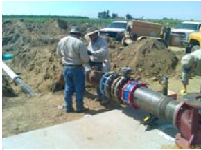
District forces make the connection from the new Turnipseed Basin recovery well to the District's distribution system.
