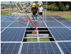
Construction of the two 30' x 40' solar panels were completed in August and September..
