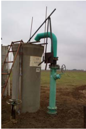
An installed float system operating a DEID turnout. The District is offering $500 rebates to the first 100 growers requesting a float system.
