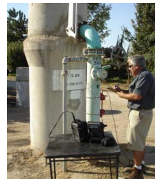
Dave Vidro from Advanced Flow Measurements calibrates a District meter in the field. DEID contracts with AFM to conduct all field testing of District meters.
